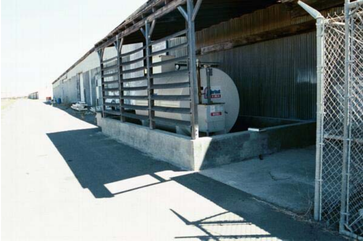
Tank A-18-1 (Diesel) - Bldg 280A
