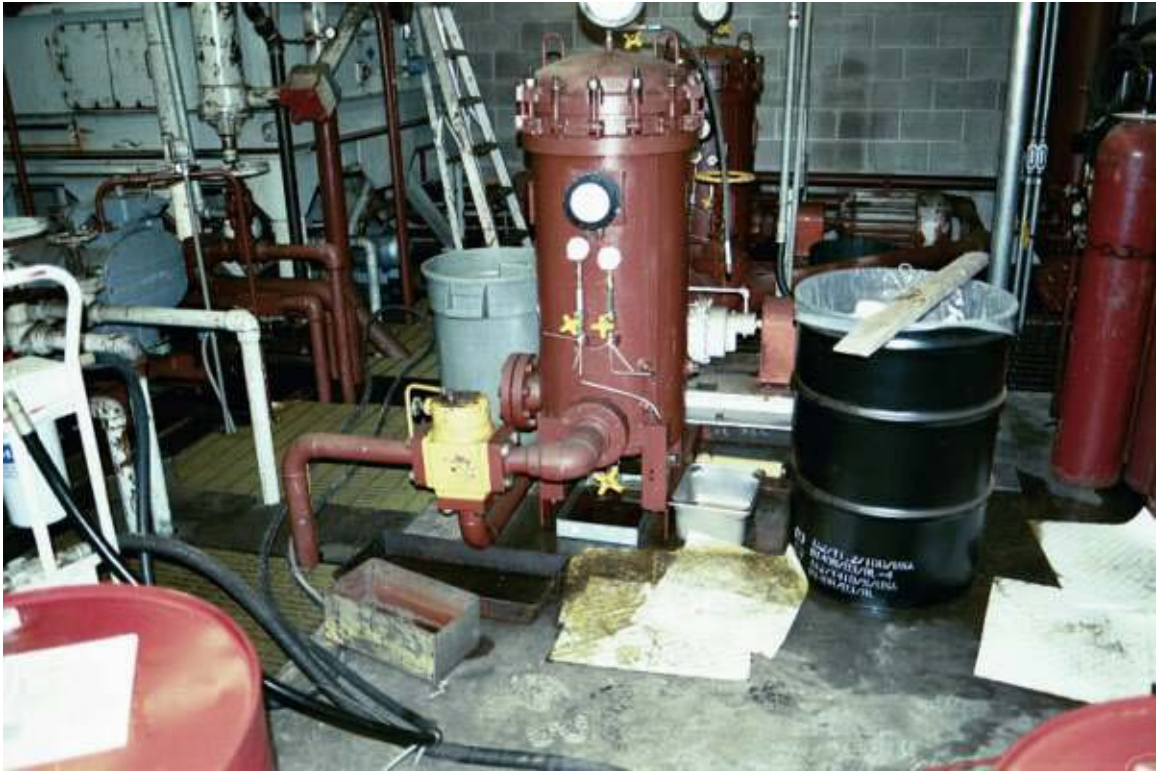
Tank A-18-3 / DSA-4 (Hydraulic Oil) - Bldg 421
