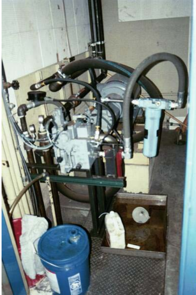
Tank A-18-4 (Hydraulic Oil) - Bldg 497
