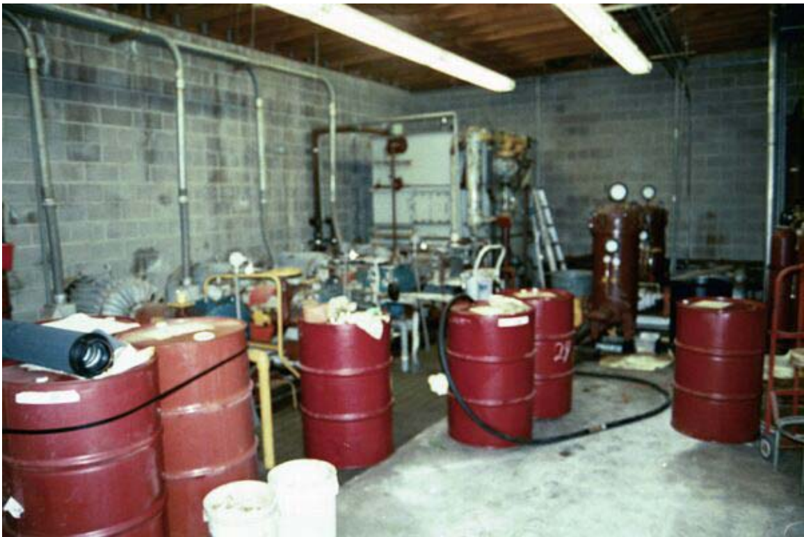
Tank A-18-3 / DSA-4 (Hydraulic Oil) - Bldg 421
