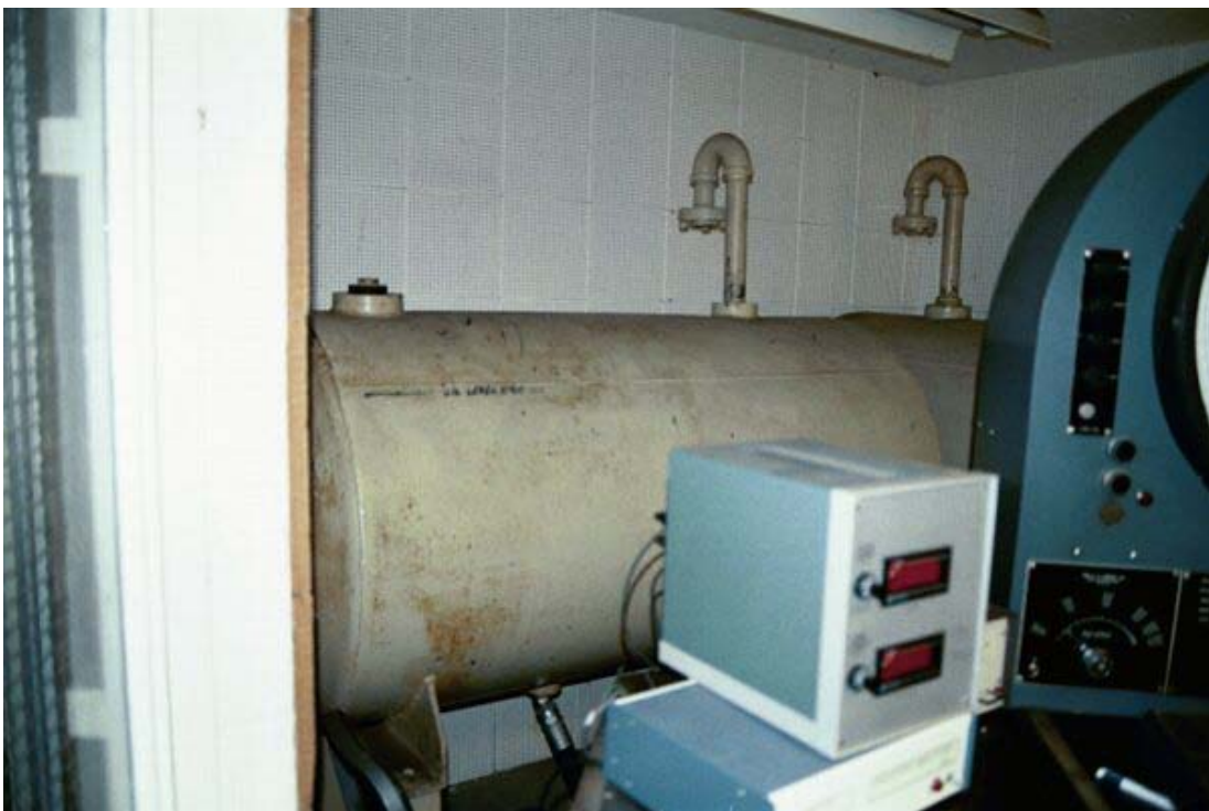
Tank A-18-4 (Hydraulic Oil) - Bldg 497
