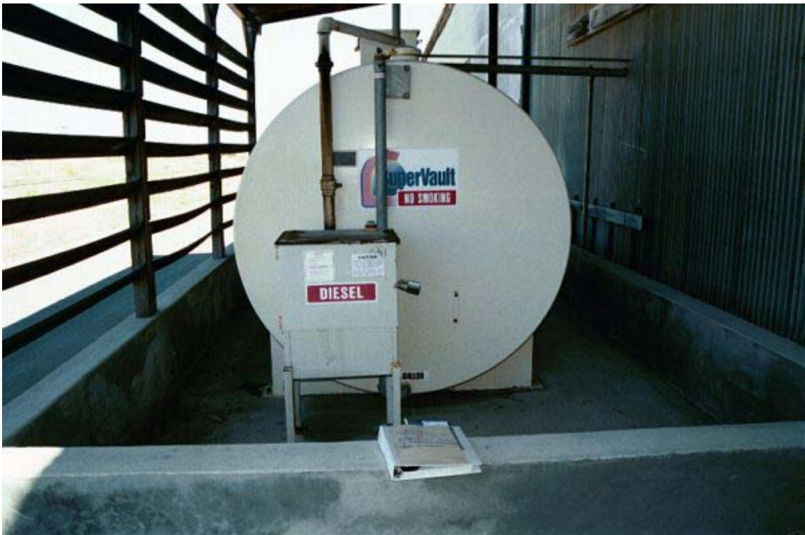
Tank A-18-1 (Diesel) - Bldg 280A
