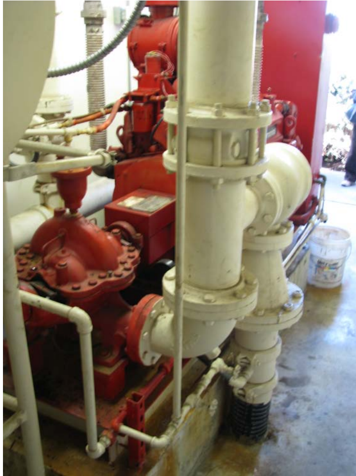
Tank A-18-5 (Diesel) - Bldg 400
