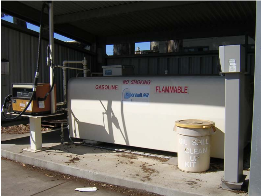
Tank A-18-2 (RFS) (Diesel) - Adjacent to Bldgs 120 and 197
