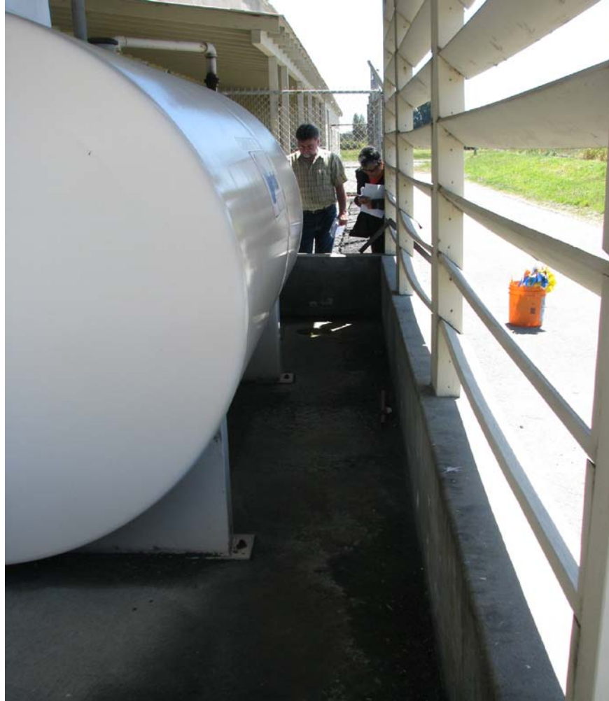
Tank A-18-1 (Diesel) – Bldg 280A
