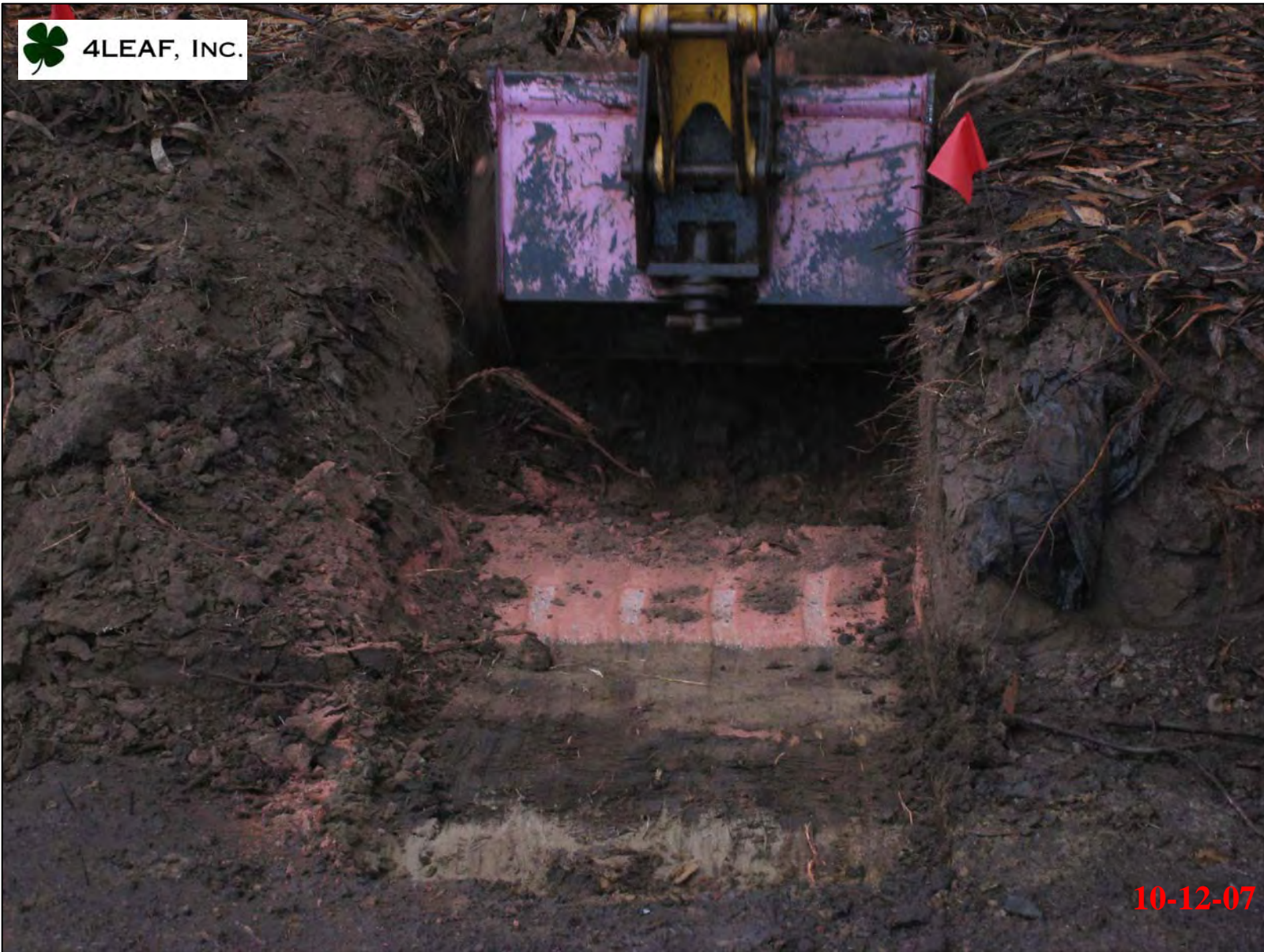
Pinkish-colored soil encountered during over excavation activities. Soil was identified as “indicator soil” for the fiber optics lines that transverse the excavation area.
