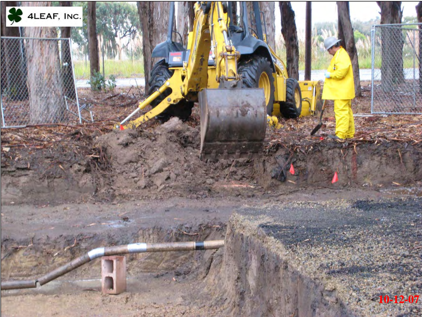
Performing over excavation in southeast portion of TCRA area after the arsenic concentrations in one of the 10/05/07 confirmation samples exceeded the project cleanup criteria.
