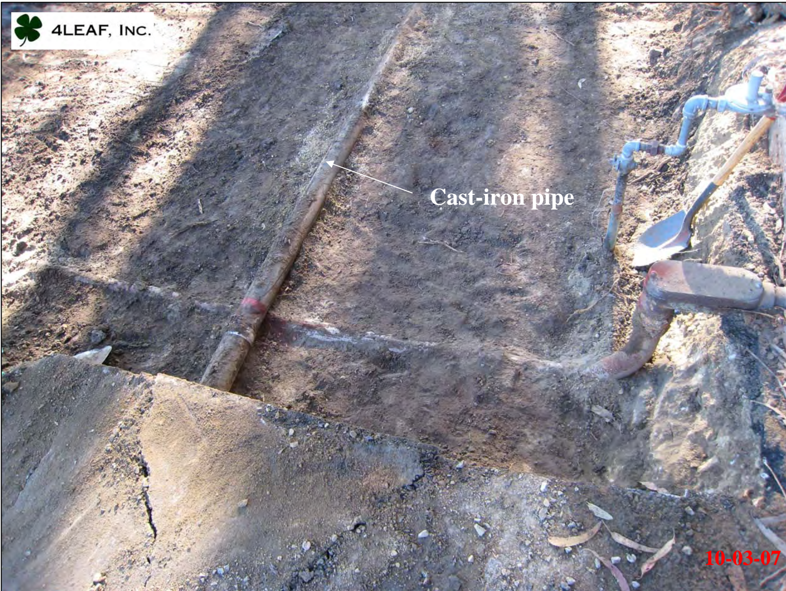
View of multiple utilities coming out of northeast corner of Building 472 in excavation area.
