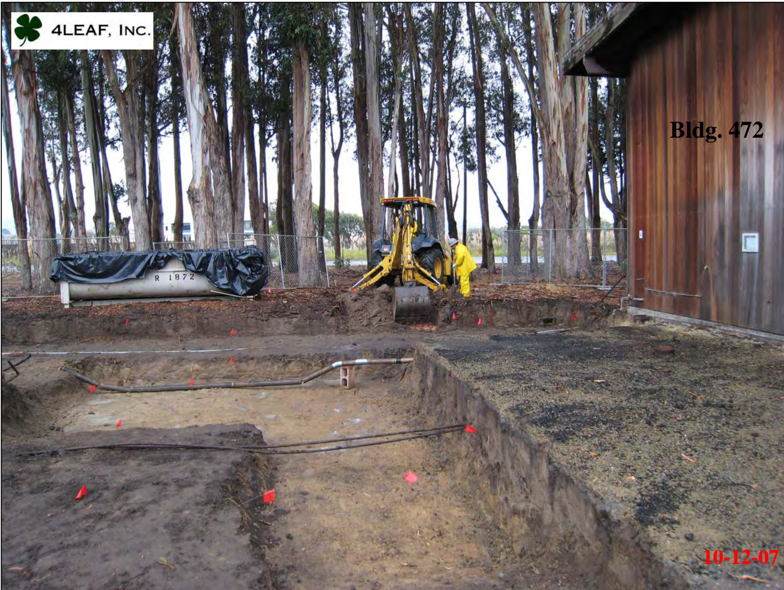
Performing over excavation in southeast portion of TCRA area after the arsenic concentrations in one of the 10/05/07 confirmation samples exceeded the project cleanup criteria.
