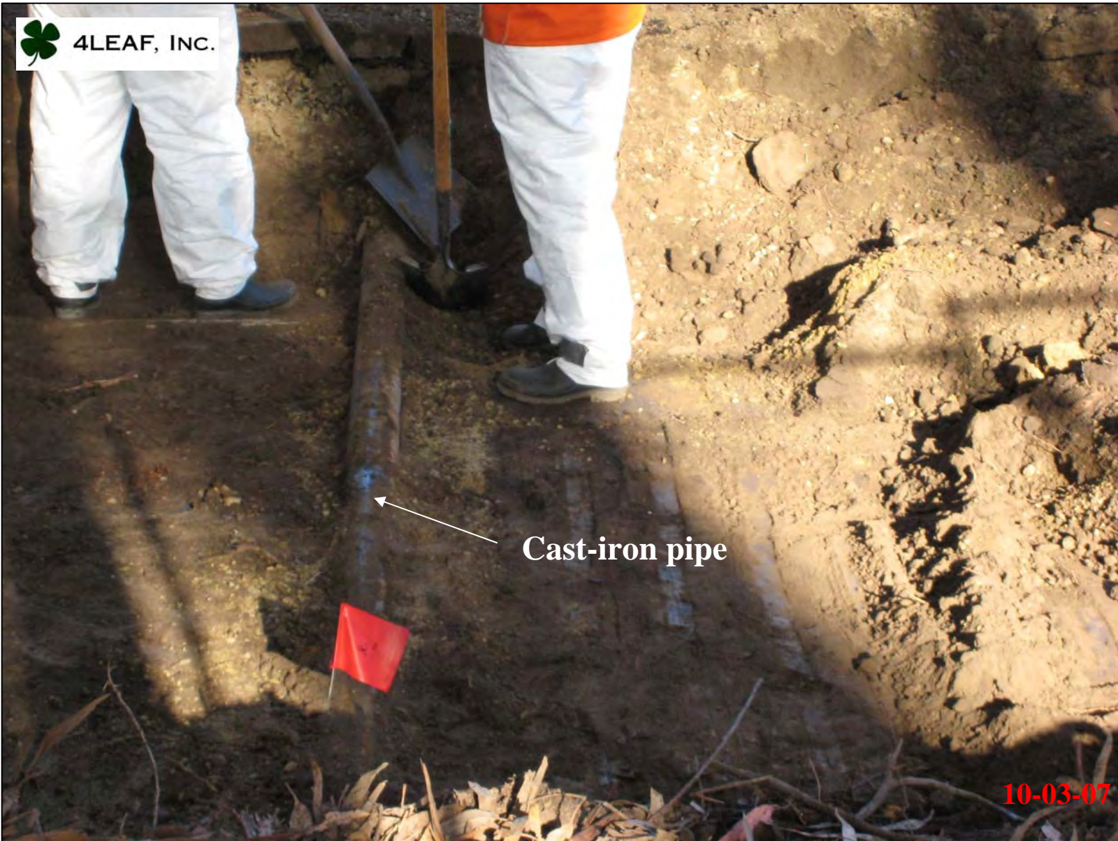
View of cast-iron pipe running in East-West direction in bottom of excavation at depth of 2 ft.
