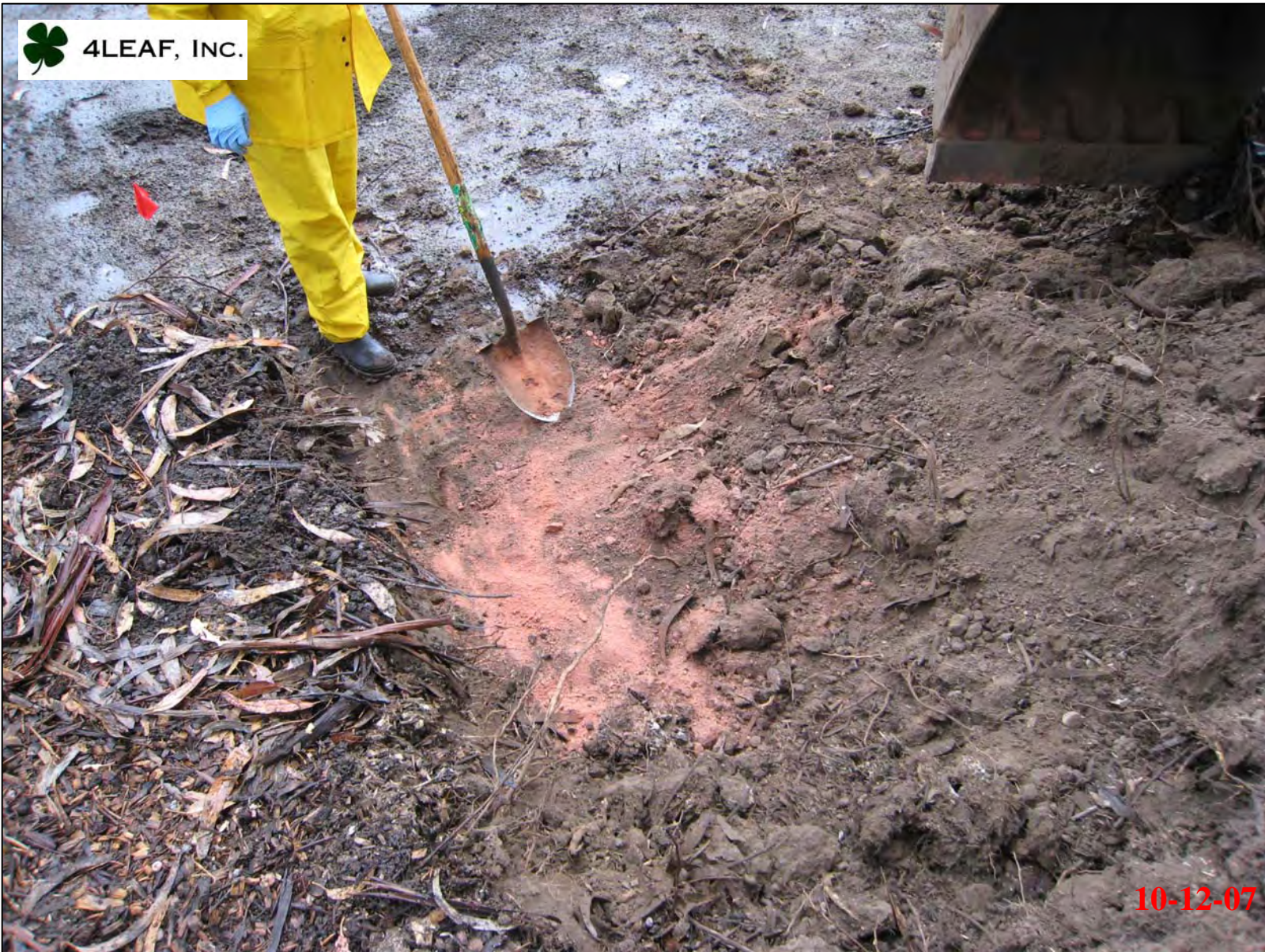
Pinkish-colored soil encountered during over excavation activities. Soil was identified as “indicator soil” for the fiber optics lines that transverse the excavation area.
