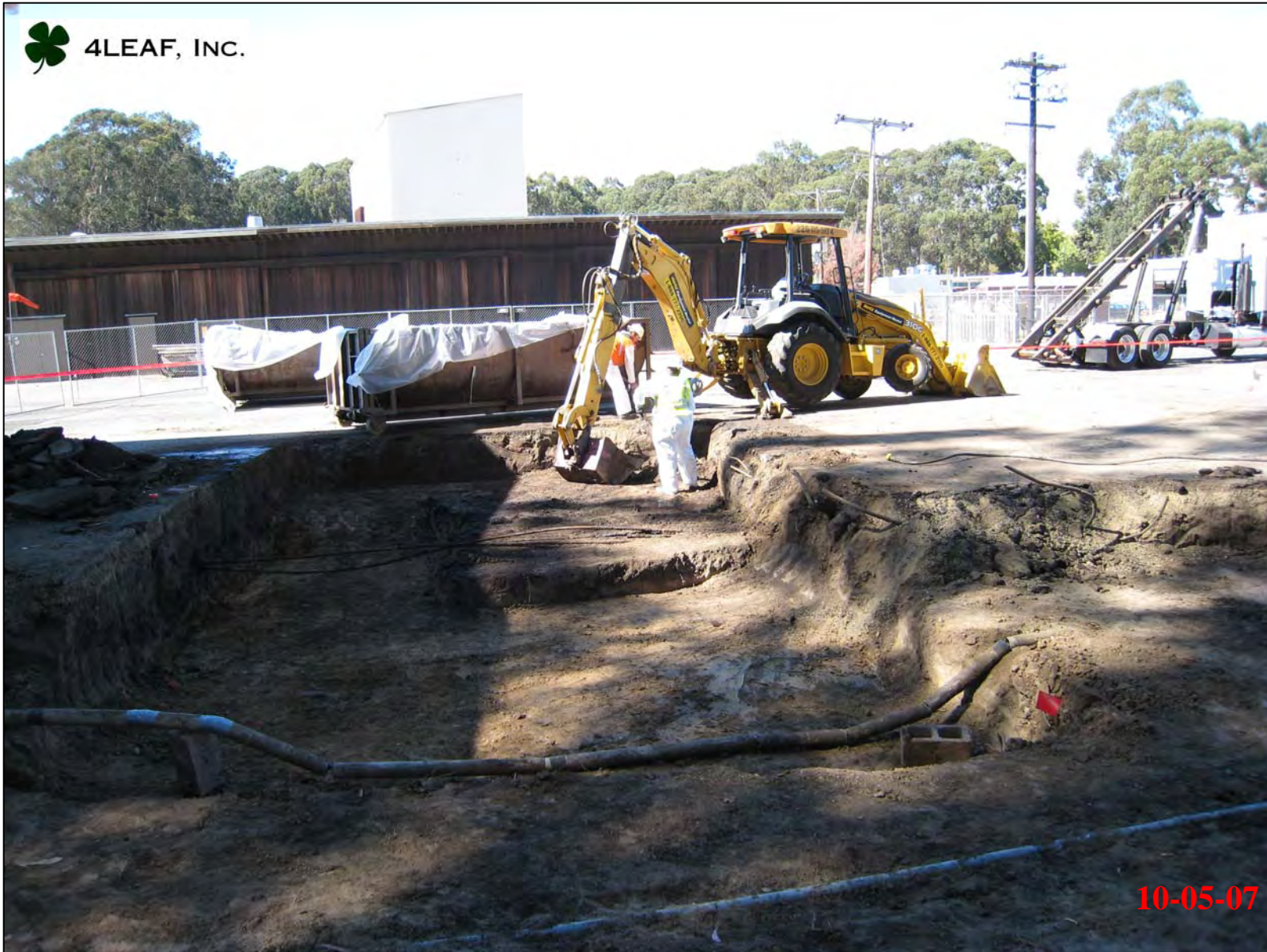
Using shovels to clean up final amounts of loose soil from excavation.
