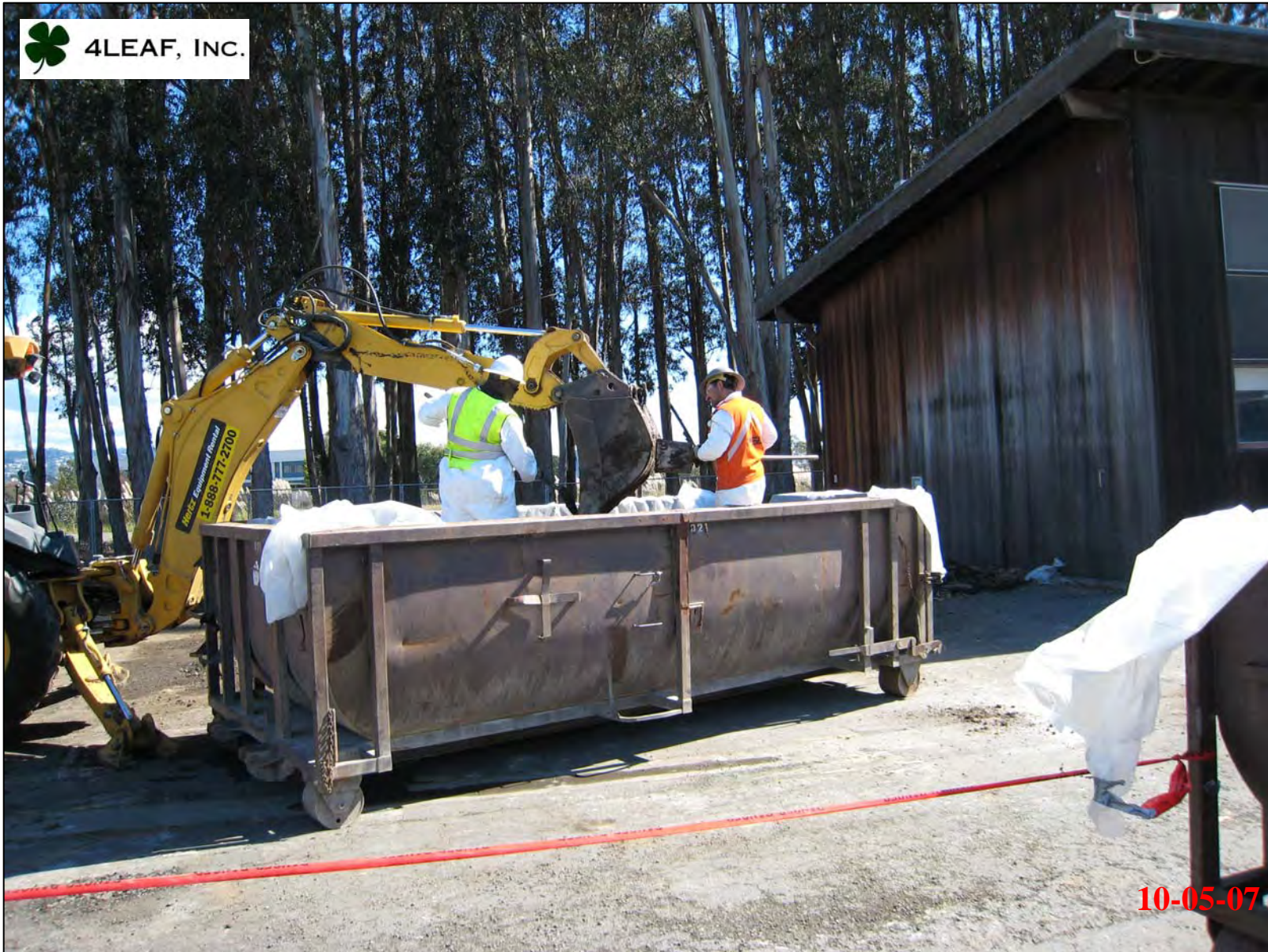
Deconning backhoe bucket using shovels to knock off loose soils into soil bin.
