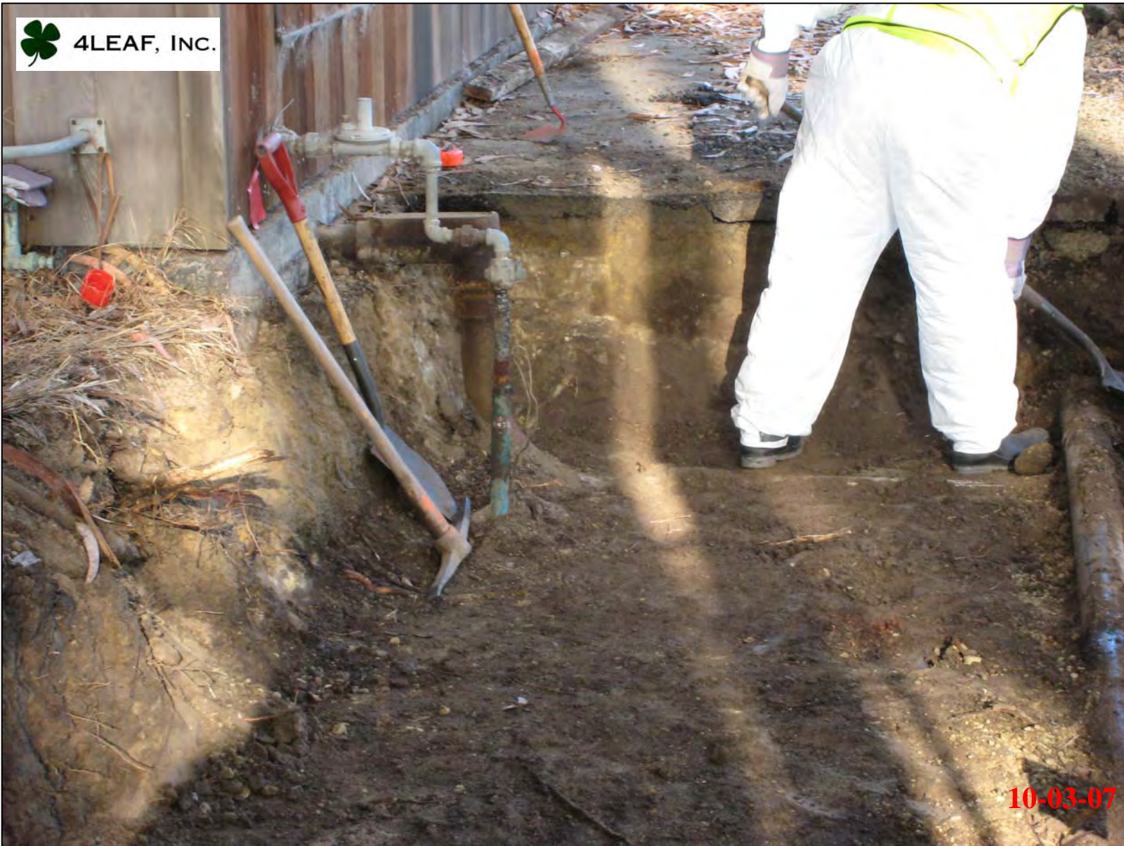
View of multiple utilities coming out of northeast corner of Building 472 in excavation area.
