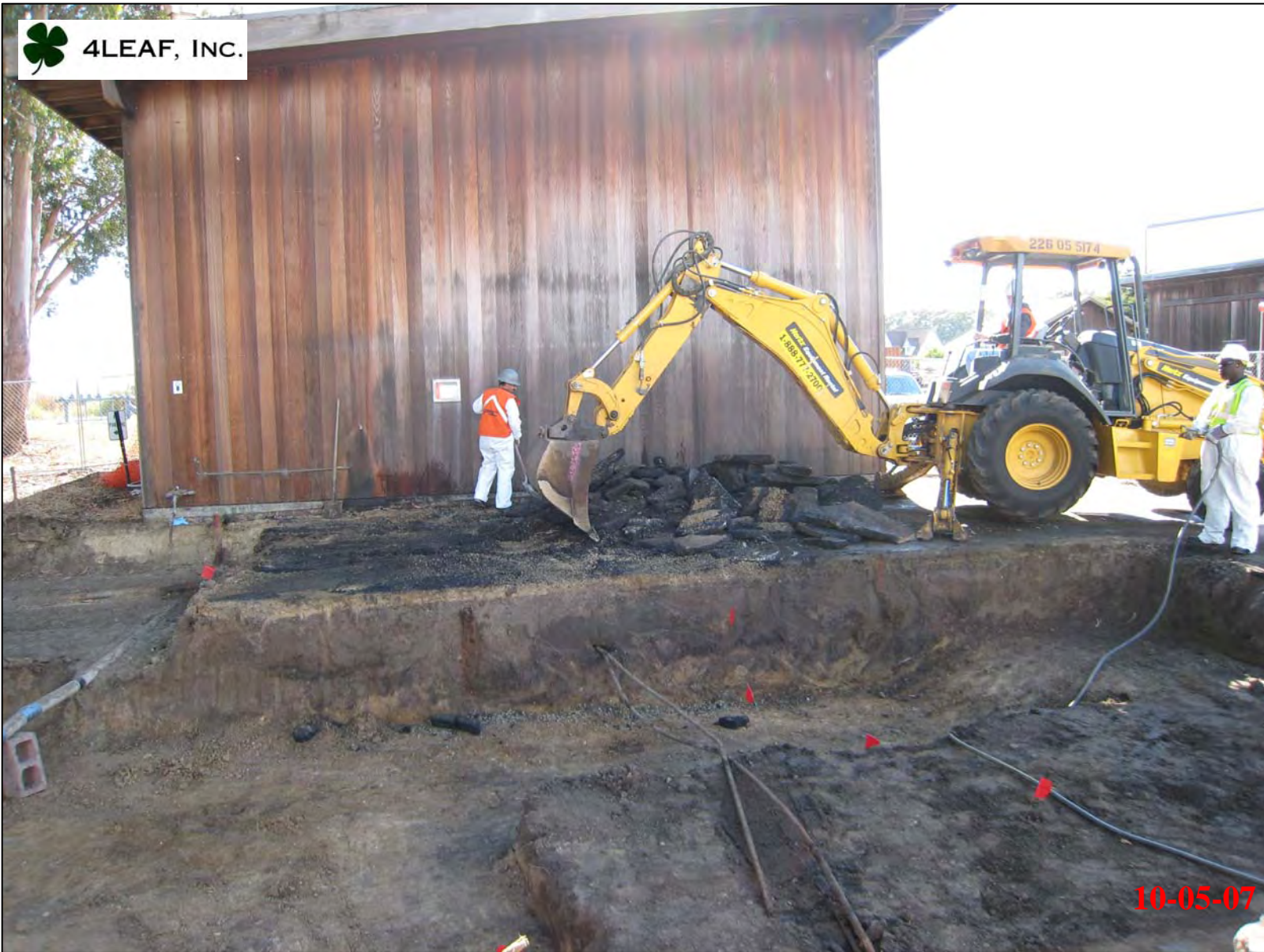
Pulling up areas of clean asphalt between north end of Building 472 and south of excavation.
